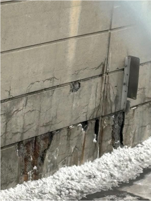
Supplemental Figure 13. Kensington Expressway, photo of Existing Retaining Walls (Beth Elkins, February 2024)
